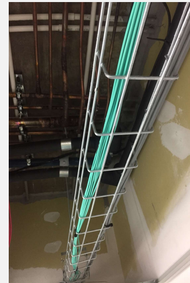
13 x Digital Theatre cabling
